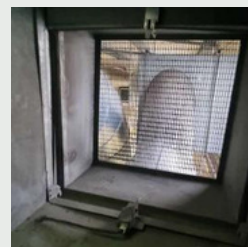
Post Test (Damper Open)
